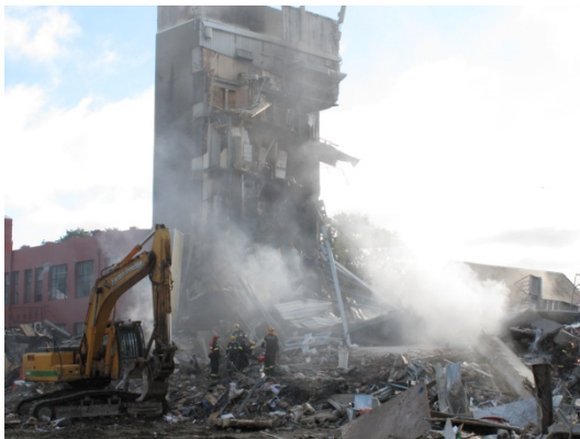
Fig.2. Canterbury Television Building
